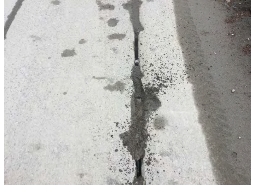
Paraseal missing and rocks edged in between slabs are causing damage
