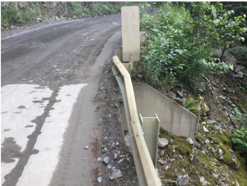
Minor damage to downstream guardrail
